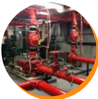
Fire Hydrant & Pump System
