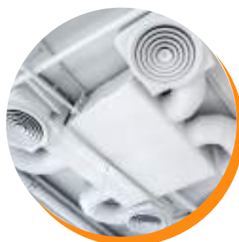
Ventilation & Air Distribution
