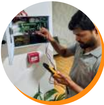
Fire Alarm System
